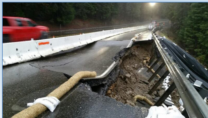
Severe Erosion on U.S Highway 50 in 2017
