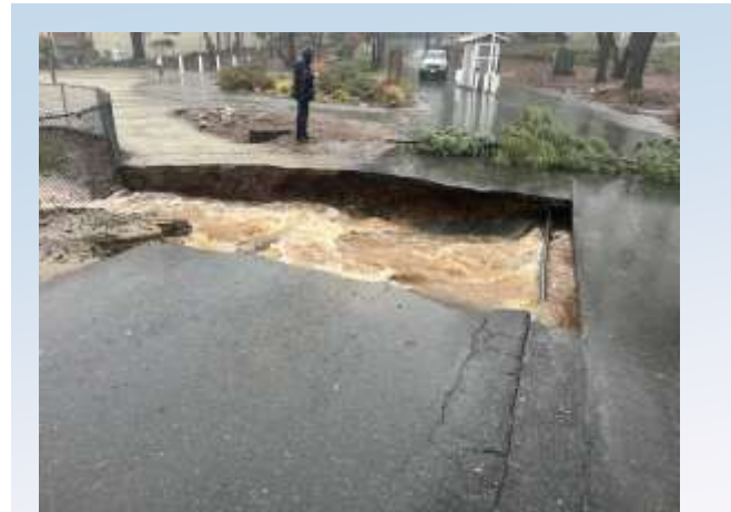
2023 Flooding in the District leading to culvert damage.
