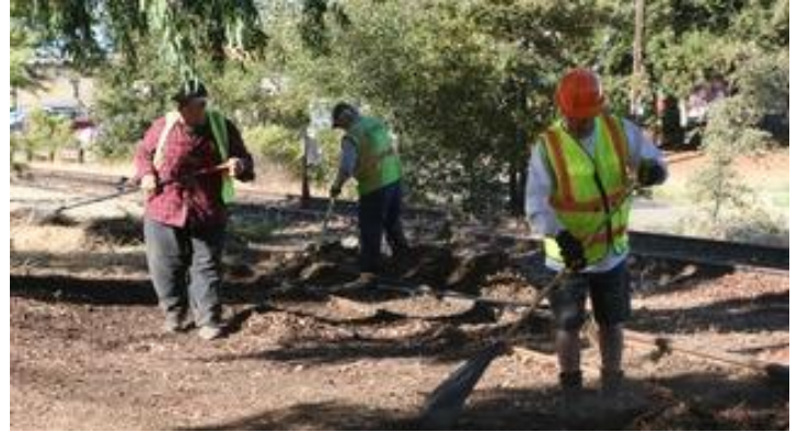
Working in the Shingle Springs yard on maintenance of way – thank you!
