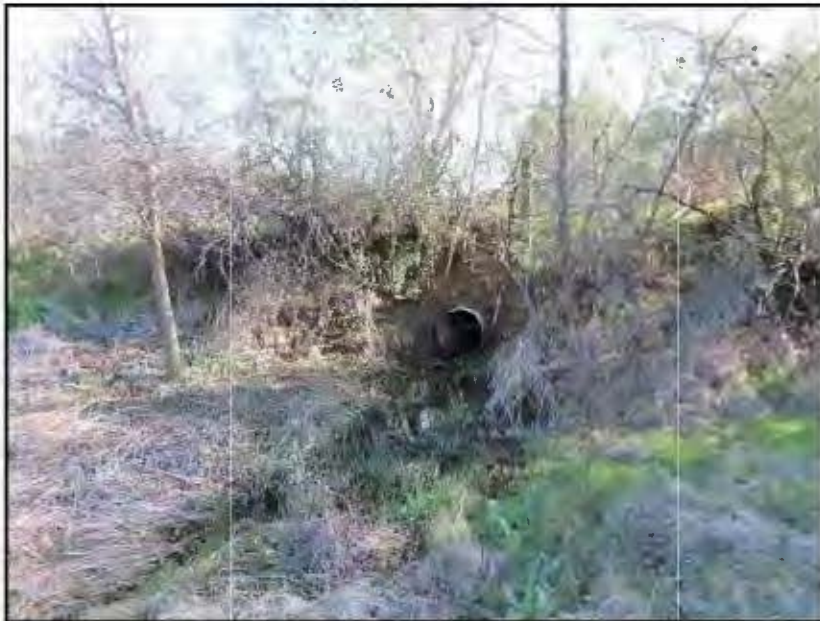
Looking south at 24" culvert under Barnett Ranch Road at southern end of property. This culvert drains Little Indian Creek swale. Photo date 2-10-21.
