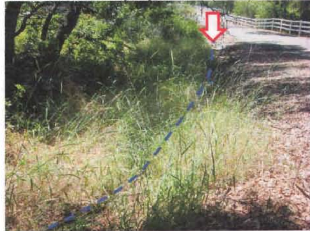
Photo 4. View looking west towards the downstream end of the ephemeral channel which flows through a culvert under Lariat Road (arrow) (28 May 2019).
