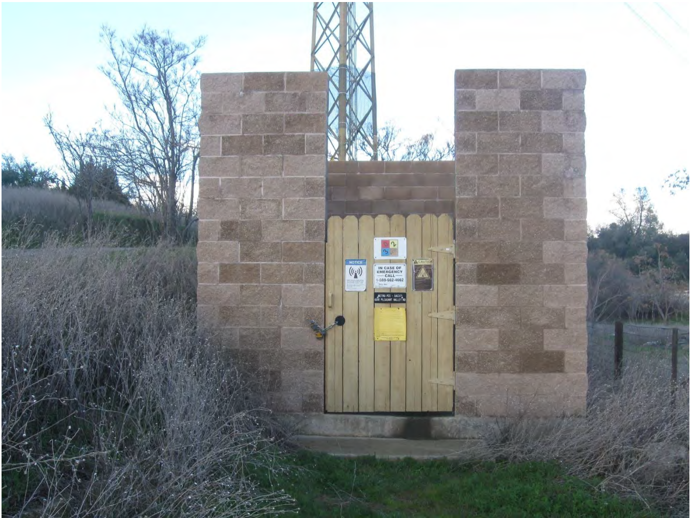
Photo showing the equipment cabinet enclosure with Knox Box lock on gate
