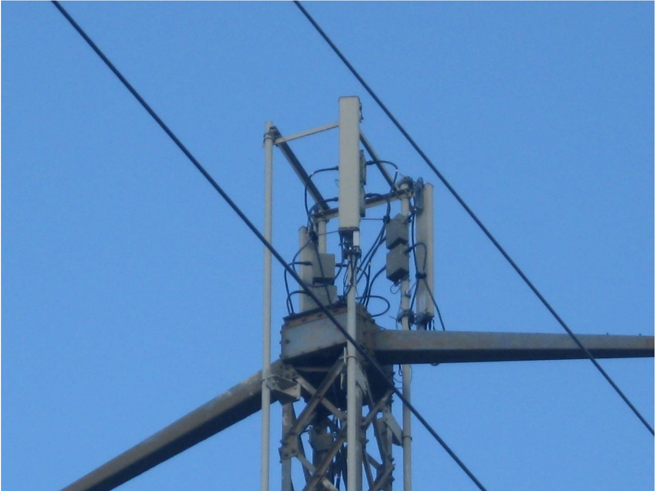
Photo showing the top of the tower with (3) installed antennas
