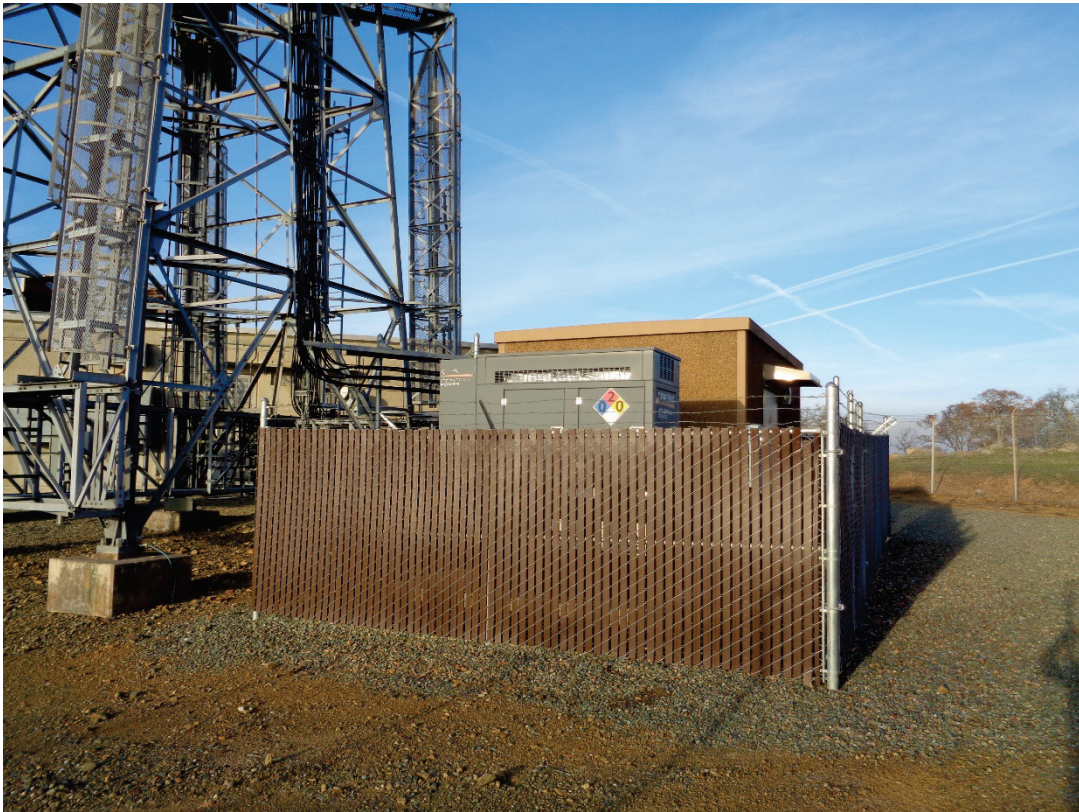
Verizon Wireless equipment shelter, surrounded by chain link fence with dark brown slats, per condition 1
