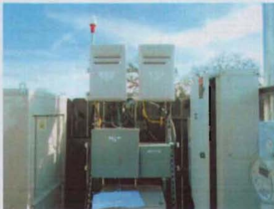
Remote Radio Units & Fiber Cabinets
