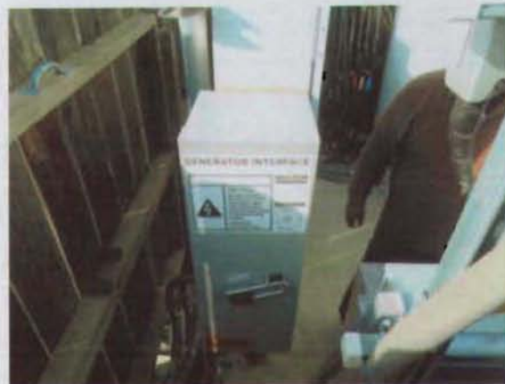
Generator Interface Cabinet
