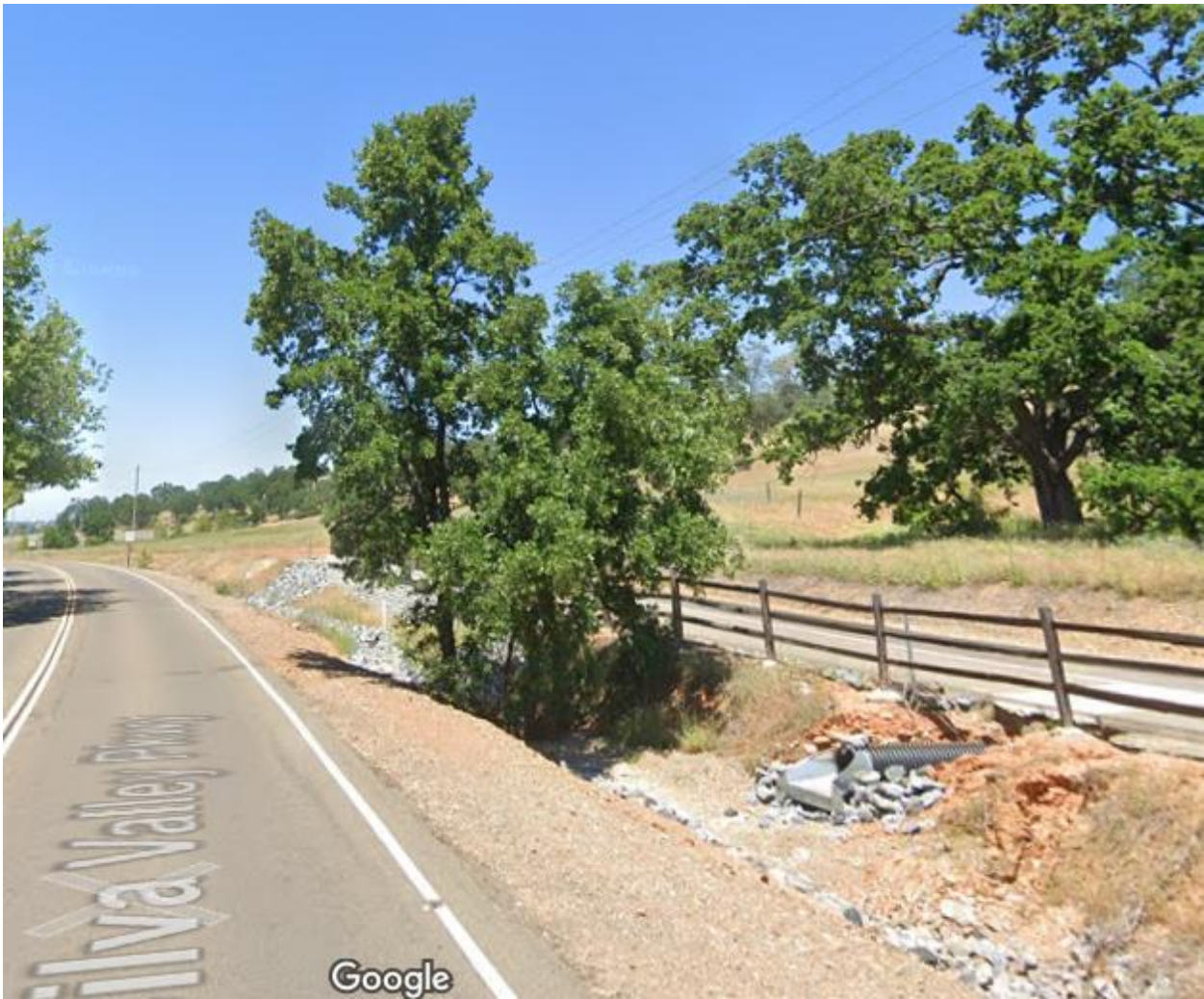
Street view of Silva Valley Parkway showing two trees growing in the drainage channel
