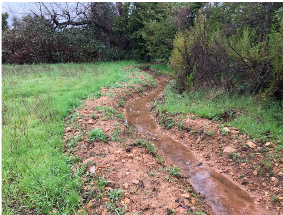
Photograph 10. Northwest-facing view of earthen swale in the northwest project area (see photograph 9).
