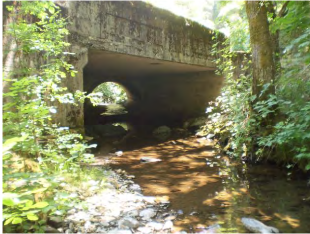
Photo 1. View east (looking upstream) toward Newtown Road Bridge over South Fork Weber Creek. 12 May 2012.
