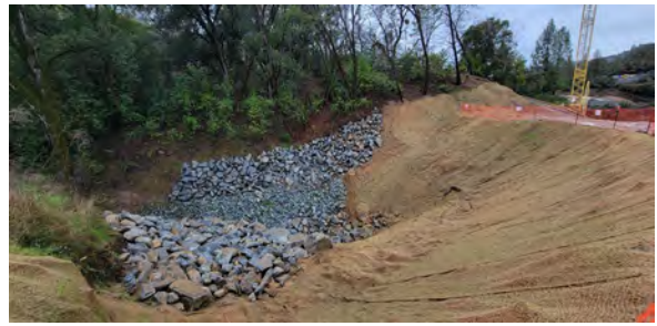
1/03/24 — DS-3/Abutment 1 Approach Erosion Control
