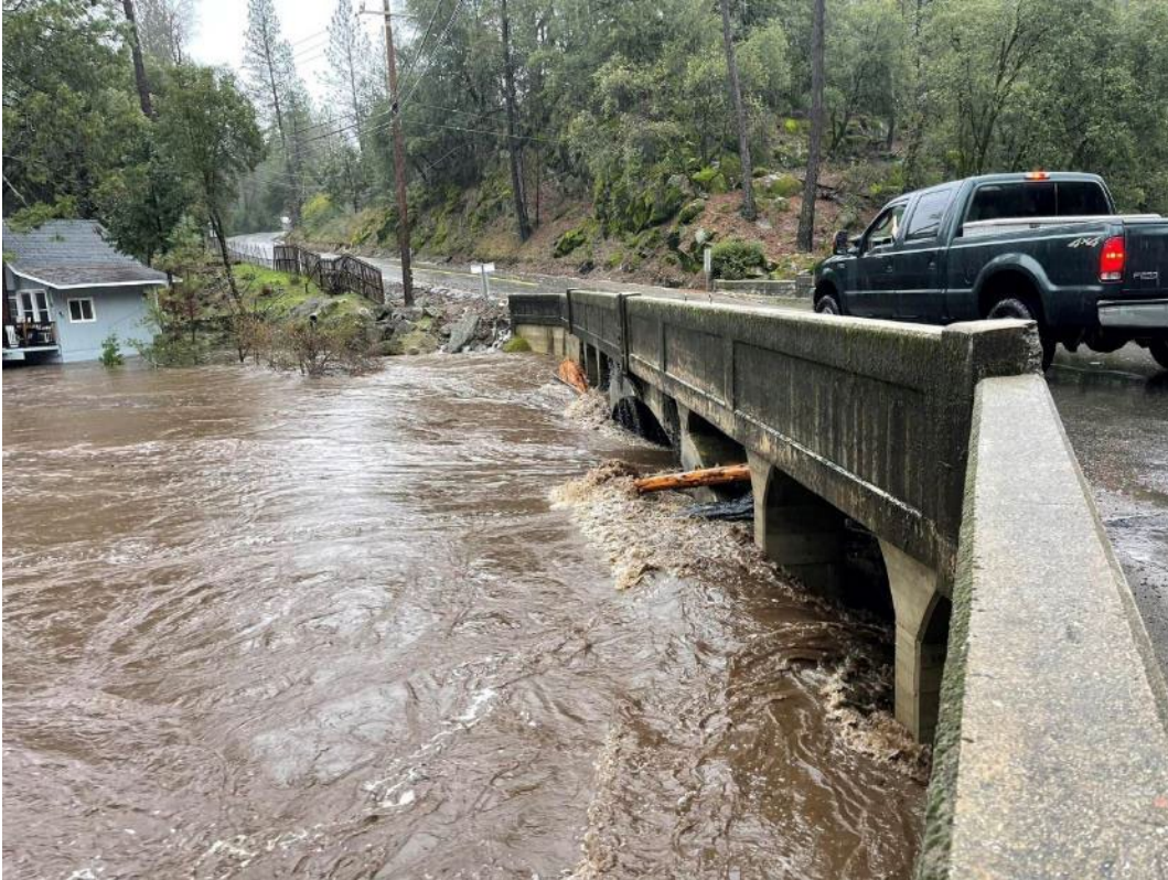
Exhibit 2-4 Bucks Bar Road December 2022 Storm Event
