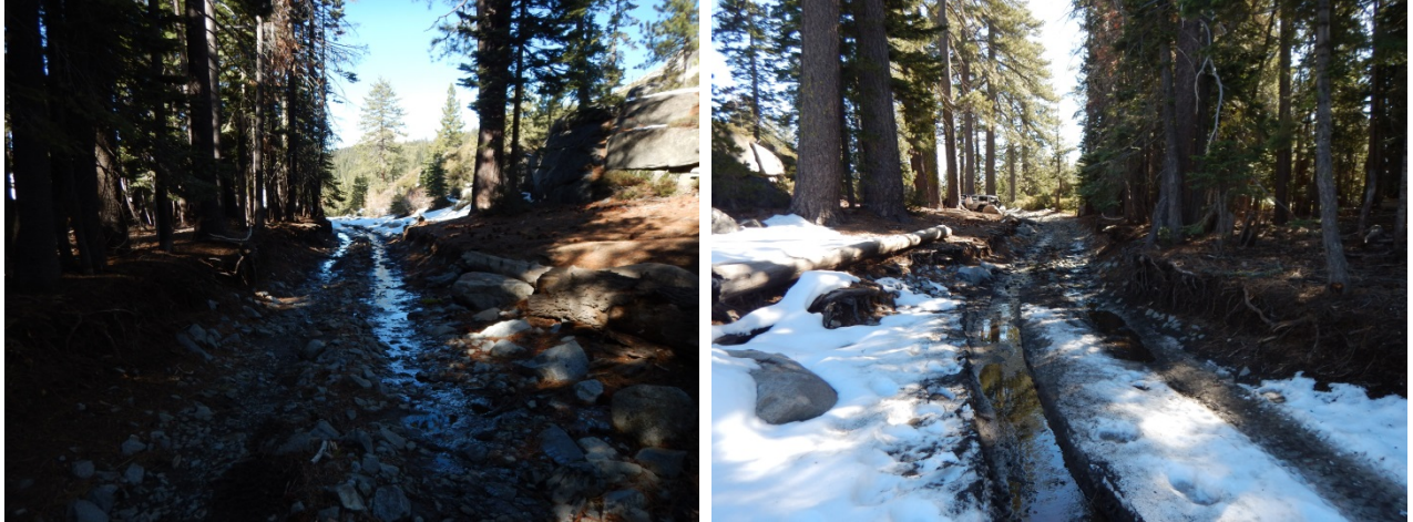
Walker Hill RT Station 165+00
