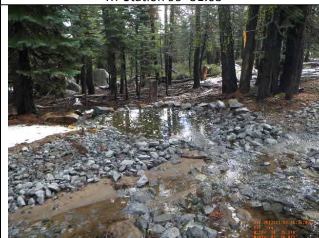
Rock Energy Dissipater RT Station 110+08.97
