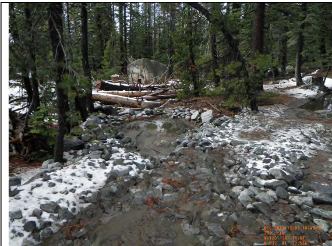
Rock Energy Dissipater RT Station 126+18.54
