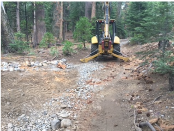
Fill on left water bar middle of picture
