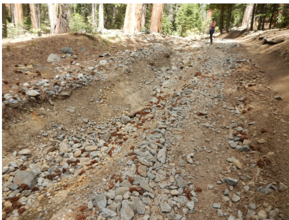
Washout 50' long x 3' wide x 3 feet deep
