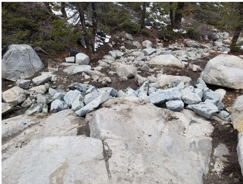
Arnolds Rock-Rock was placed to make it easier for the pumper truck
