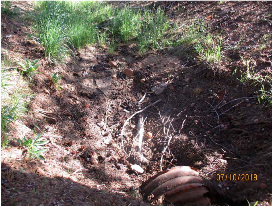
Photo 3: Culvert 1a, C1a, looking north at the north side of the road (downstream).
