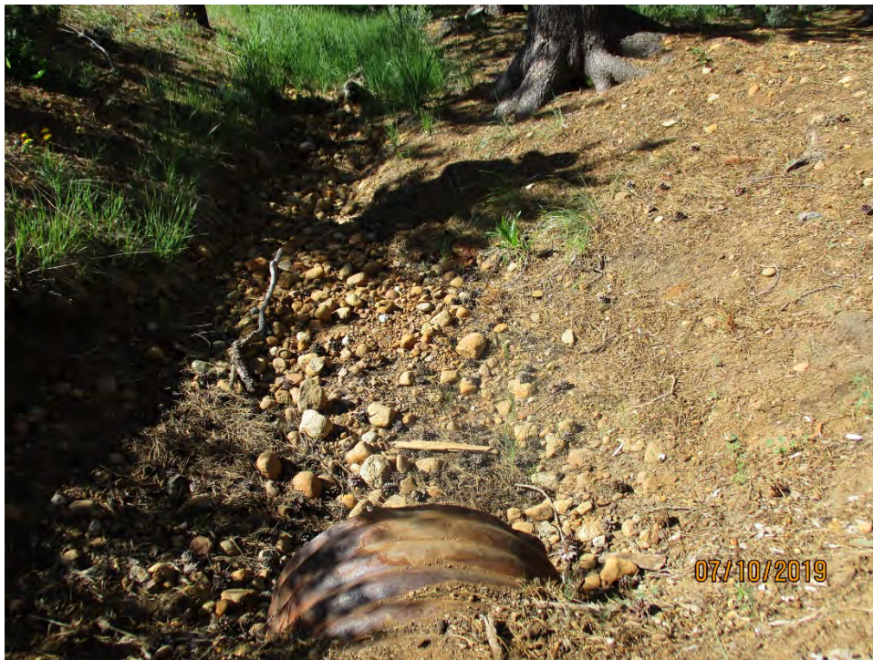
Photo 4: Culvert 1b, C1b, looking south at the south side of the road (upstream).
