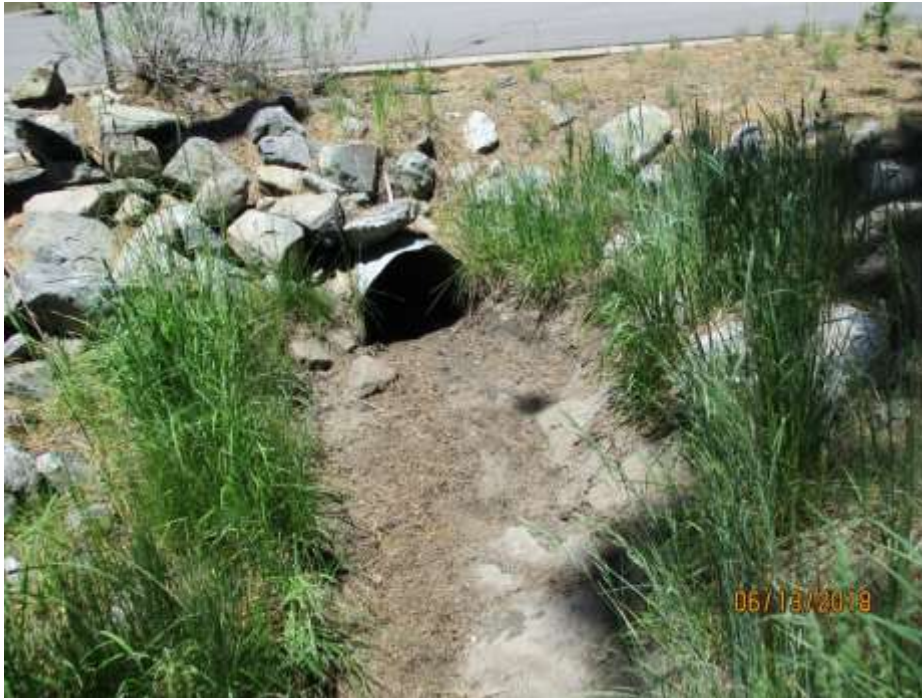
Photo 9: Isolated Unnamed Drainage 3, upstream of Data Point ISO 3, looking upstream at culvert.
