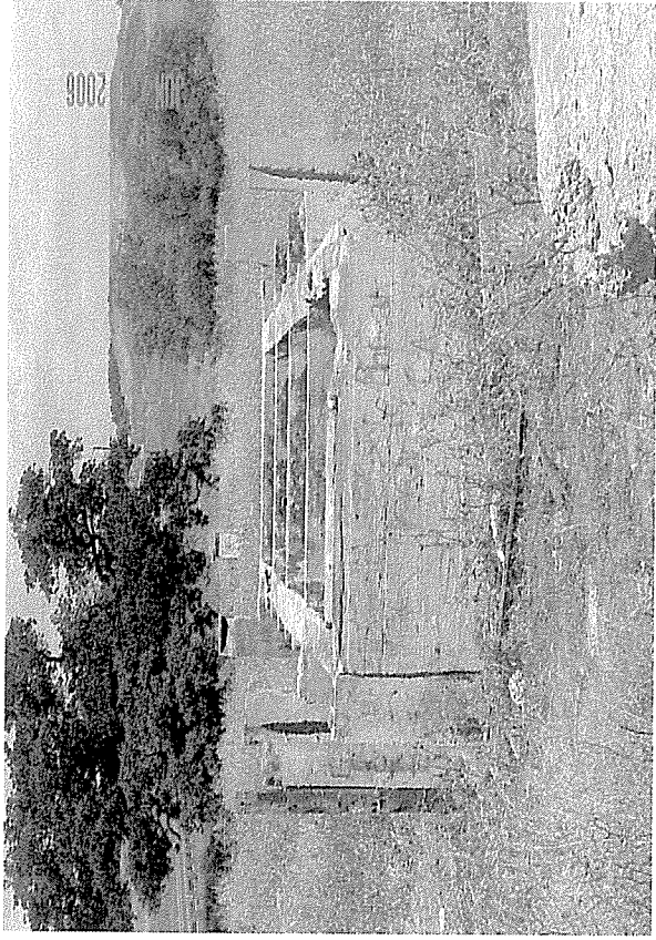
Photo 42: Lot 1; close-up of the "basin" structure. Looking north. Silva Valley Parkway can be seen on the left.
