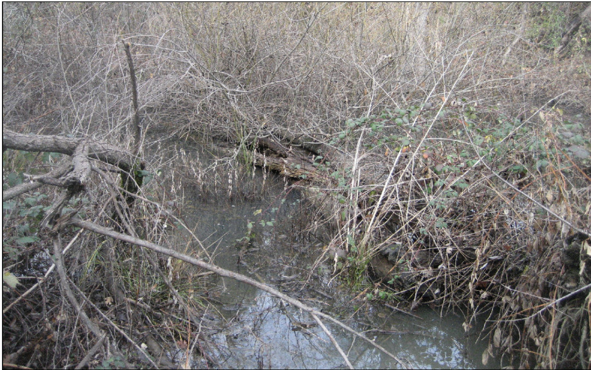
Photograph 5: View of outlet of Ephemeral Drainage 4 (ED4). Shows culvert beneath dirt road that discharges water into wooded area in the northern portion of the Project Site. Photograph taken January 8, 2008.
