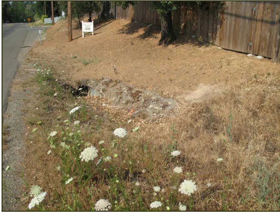
Photograph 5. Photograph of roadside ditch (RD3) and culvert located on the north side of Pleasant Valley Road near Ryan Drive. Photograph taken just east of the feature looking southwest along Pleasant Valley Road.
